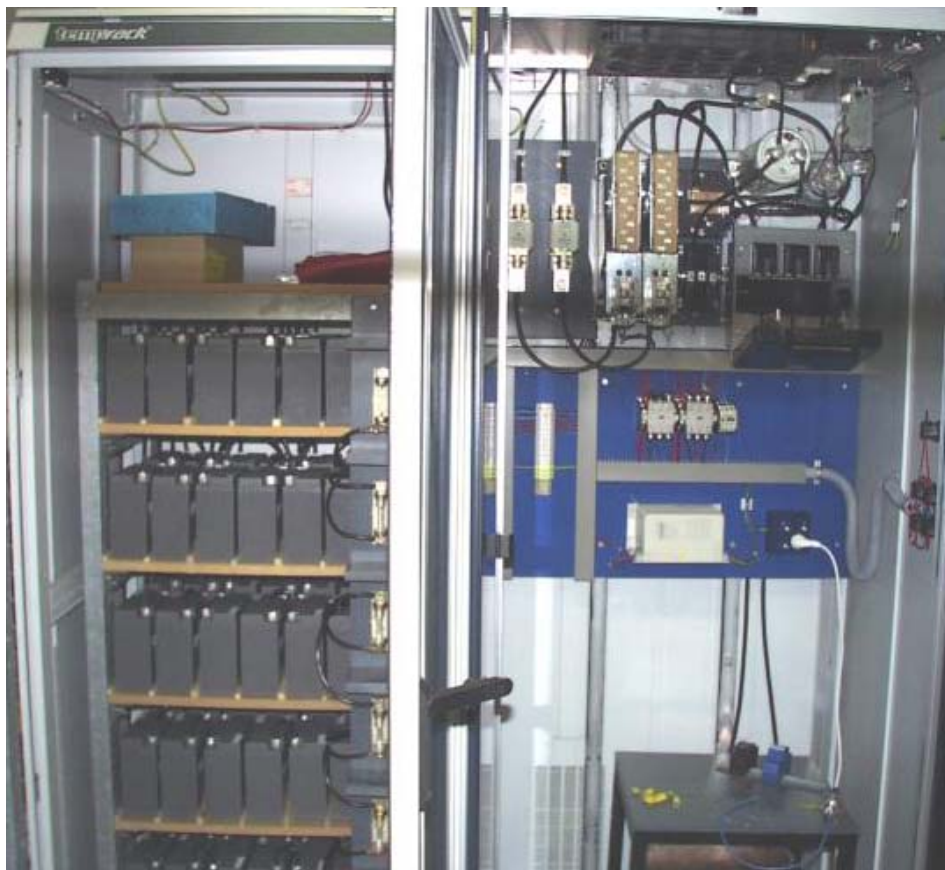
Fig.8 Long duration DC-Generator for 870 volt and 500 A.
