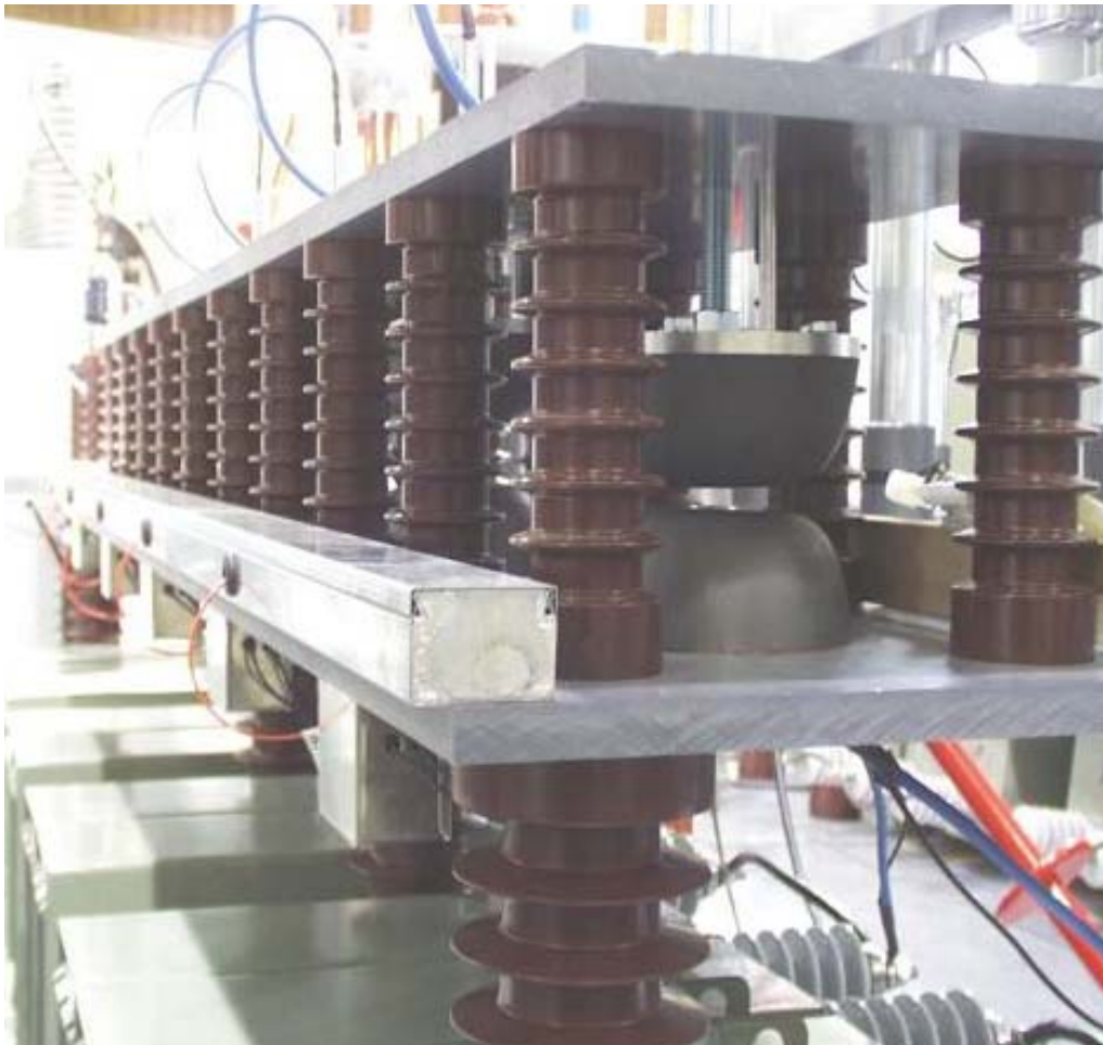
Fig.6 view of one part of the generator containing 5 stages.
